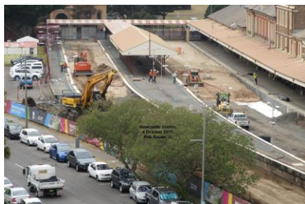
Filling in vacated track space at Newcastle Station in 2017. Source: Bob Rouse.
