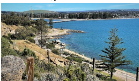
Engineering works in progress along where the horse drawn tramline runs...public not able to access this area at present.
