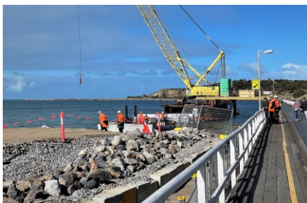
The new Granite Island Causeway engineering job was 3 months in progress when this photo was taken on May 14 th , 2021. The location is at the Victor Harbor end and foundation work was in progress, but no causeway structure. (This photo and others can be seen in the July 2021 TTGGMC Newsletter, page 9, column 3.)
