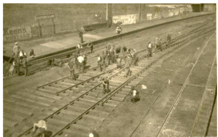
Laying in new rails and sleepers at SMR's East Greta Junction. Source: Mal Austin .
