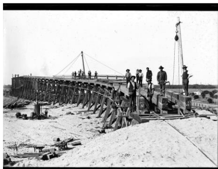
Constructing Port Waratah Coal Stage in the days of block and tackle. Source: Flickr.
