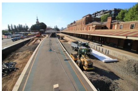
Ripping up the 1858 rail extension to the heart of Newcastle in 2017. Source: Railpage .
