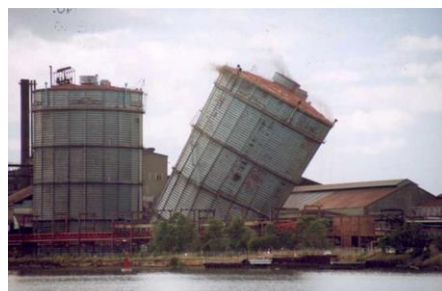
A gas holder coming down during demolition at BHP Newcastle's Steelworks. Source: NIHA.
