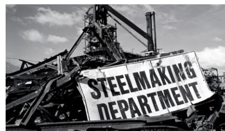
The end of steelmaking at Newcastle as the plant is demolished. Source: Central Western Daily.
