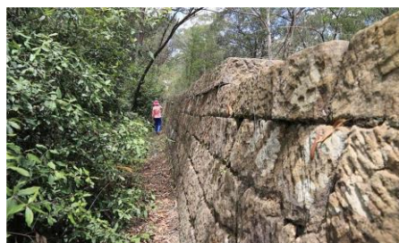
A convict-built stone embankment on the Great Northern Road still revealing the chain gangs' pick marks. Source: Stephen Gard.
