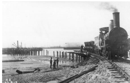
BHP Locomotive No.1. "Old Lizzie" hard at work with the Steelworks construction in 1913. Source: NIHA.
