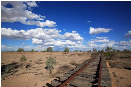
Flood-ravaged remnants of the Great Western Railway to Bourke. Source: Railpage - DMB Photography
