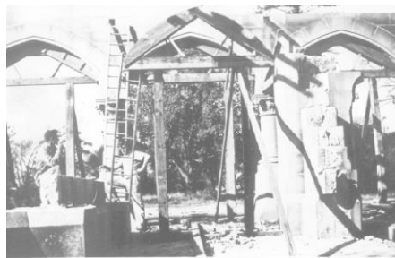
During the demolition in 1958 each stone was marked and added to the architectural plans. Source: ABC Canberra .
