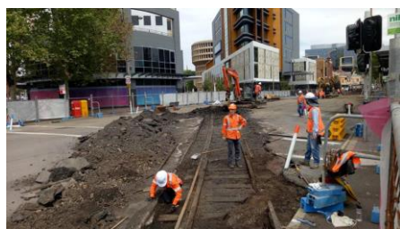
Newcastle workmen unearthing a tramway and railway line from the 19 th century. Source: Newcastle Live.
