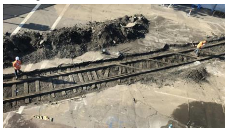
Burwood Line railway track exposed with dual diagonal tram line crossing inserts in Hunter Street. Source: Newcastle Live.
